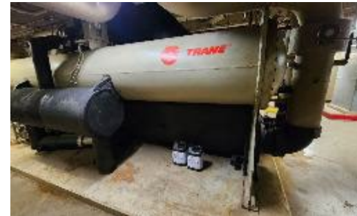
Main chillers for building in need of replacement.
