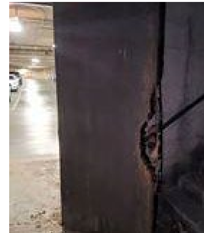
Corroded interior door of parking garage interior stairwell
