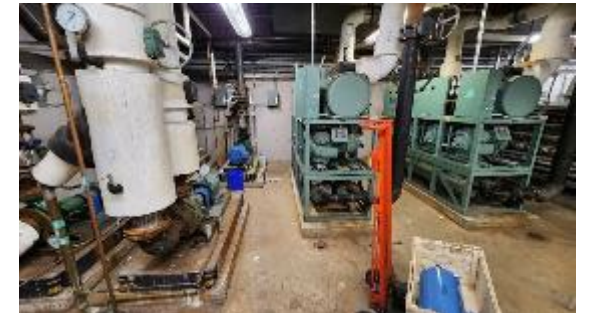
Back-up chillers for the data center in need of replacement.
