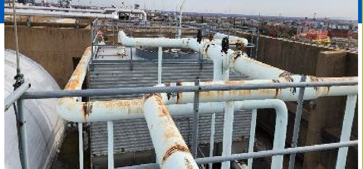
Corrosion visible to original condenser water piping (at roof).
