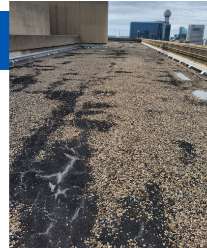
Typical condition of roof membrane, exhibiting widespread surface deterioration and nearing end of typical service life.
