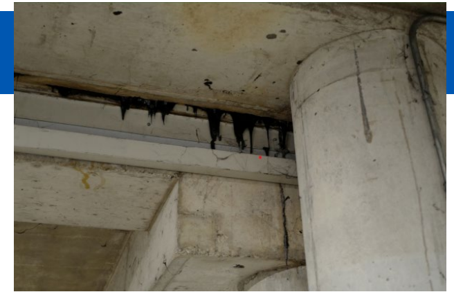
Coal tar pitch dripping at expansion joint directly above the gutter system installed to capture leaking water
