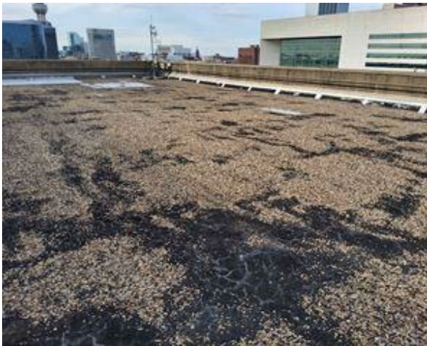
Deteriorated Roof Membrane
