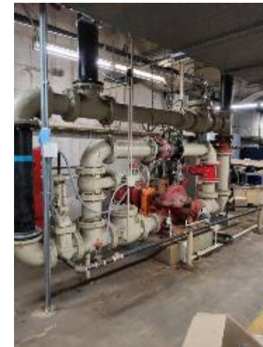
Fire suppression wet system
