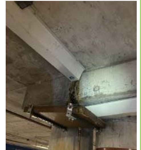
Signs of water intrusion in parking garage.
