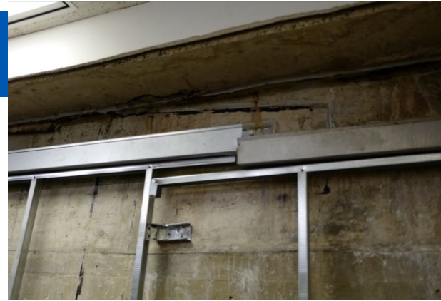
Example of gutter system to capture leaking water at IT space within building interior
