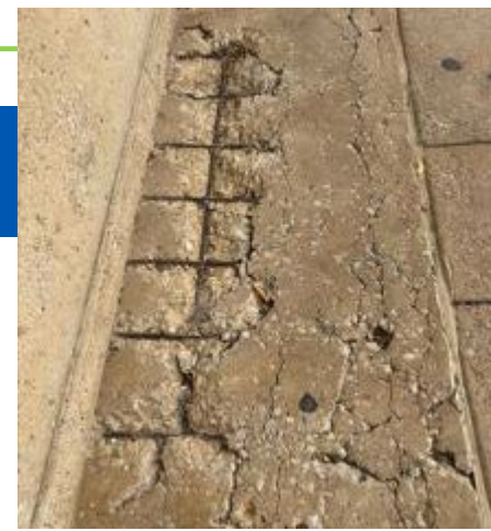
Spalled concrete with exposed reinforcement observed at City Hall slab edge, indicating localized structural deterioration.
